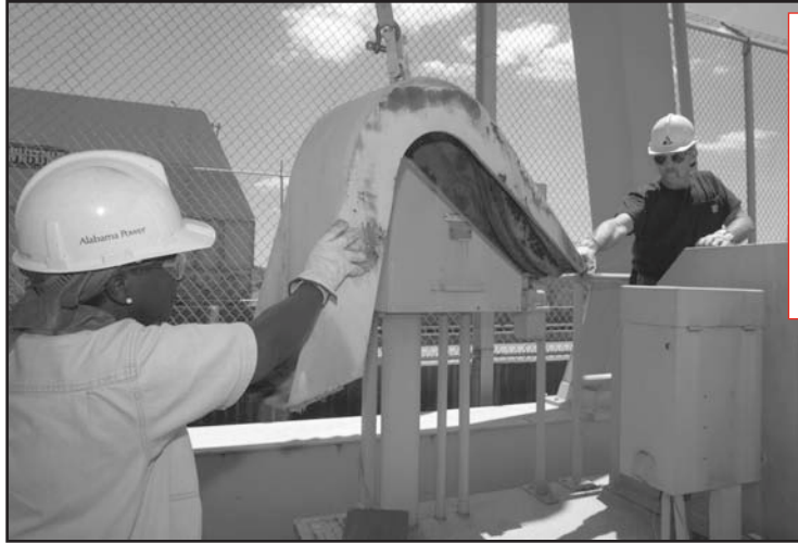
CAREFUL, CAREFUL ... KATIE GLENN (LEFT) AND PAUL POOLE REMOVE HEAVY METAL GEARBOX COVERS FROM THE MOTORS THAT OPERATE THE SPILLWAY GATE CHAIN AT NEELY HENRY DAM.
